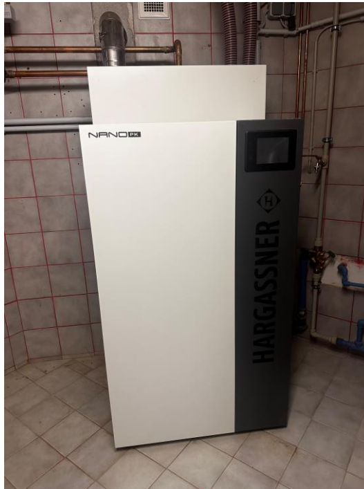
Figure 8: The new pellet boiler of the example household
