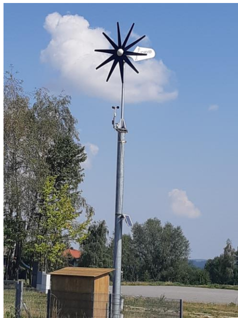
Figure 48: The small wind turbine of the brand Schachner, SW1.5, installed in Großschönau
