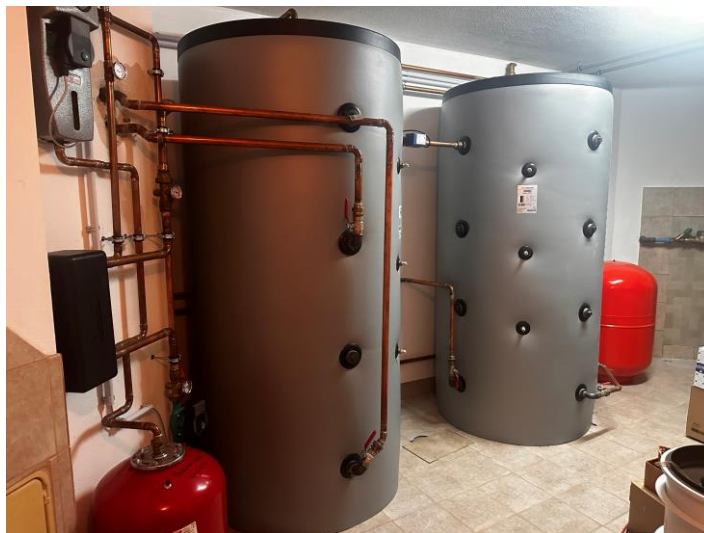
Figure 9: The two buffer storage tanks of the example household
