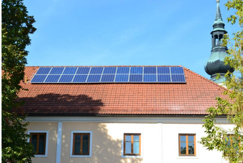
Figure 47: Current PV-system on the municipal office and potential roof area for a further installation
