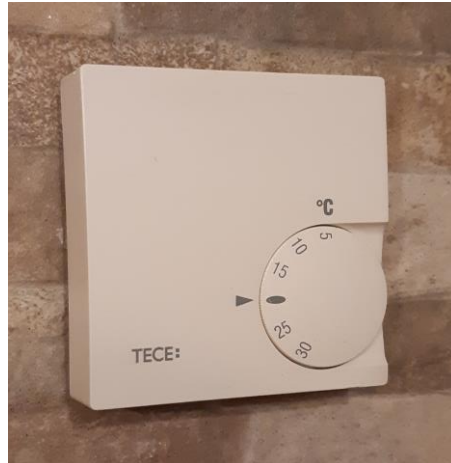
Figure 7: Room thermostat for adapting the temperature to the usage of the room
