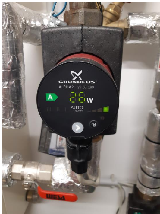
Figure 5: An example of a high-efficiency DHW pump in Großschönau
