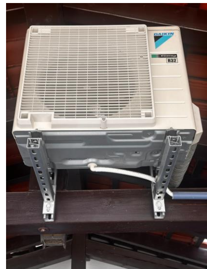
Figure 11: Example air conditioner – outdoor unit
