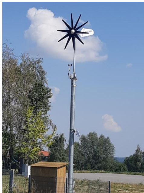
Figure 48: The small wind turbine of the brand Schachner, SW1.5, installed in Großschönau
