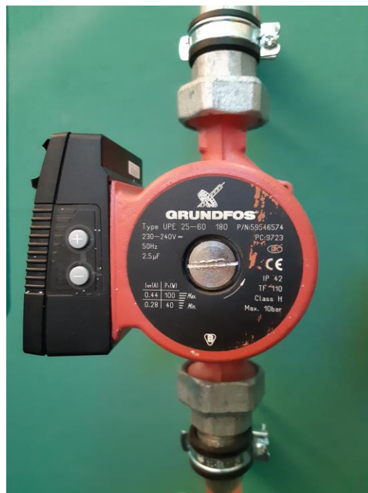
Figure 6: An example for an old DHW pump in Großschönau
