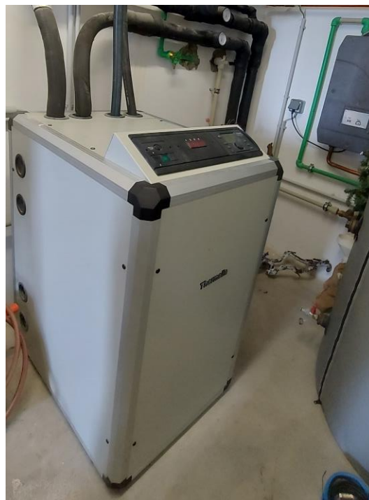
Figure 4: Heat pump of the brand Hoval, Thermalia R 7P
